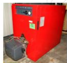
Reference: BLY-026 HEATING BOILER Year: 1997 Brand: Savio Width: .
