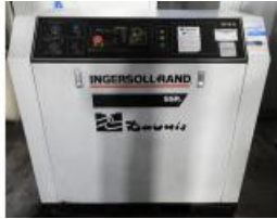
Reference: CTB-157A AIR COMPRESSOR 18.5KW Year: 1998 Brand: Ingersollrand Width: .
