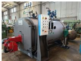
Reference: AV7-014 STEAM BOILER 1750kg Year: 2016 Brand: PERELLÓ I.VAR Width: .
