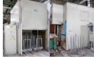
Reference: LAN-110 Dryer (Bobines) Year: 1998 Brand: Galvanin Width: 0
