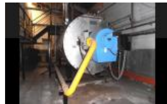
Reference: TIG-01 STEAM BOILER Year: 2000 Brand: Steambloc Width: .
