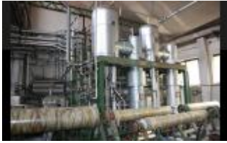
Reference: LUI-037 Cooling and Recuperator for Ca... Year: 1987 Brand: Kasag Width: -
