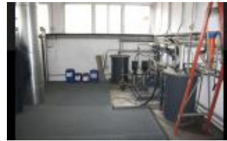
Reference: LUI-082 Osmosis System Year: 1998 Brand: Babcock Wanson Width: -
